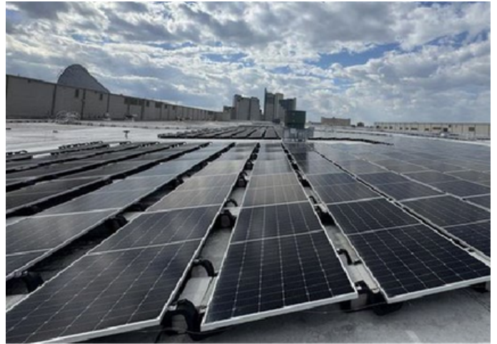
Newsolar array at the Orange County Convention Center
