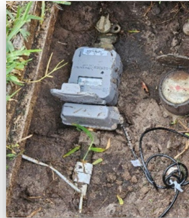
An example of the in-ground residential ultrasonic water meter
