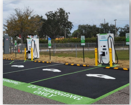
DC Fast-Chargers at East Orange Community Center
